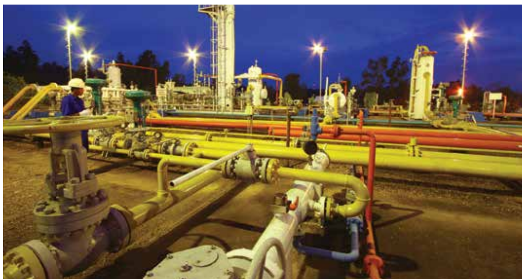
Gas Gathering Station - Medco E&P
