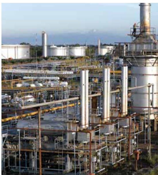
Gas Plant - VICO
