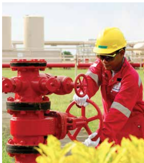
Wellhead - Kangean Energy
